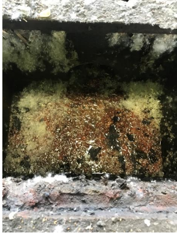
Figure 9. CB6 with lid removed.
