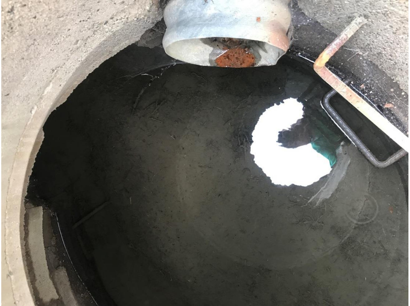
Figure 3. CB3 with the lid off revealing the artificial stream bed. Sediment depth is \geq 18'' . The metal pipe discharges stormwater from CB7.
