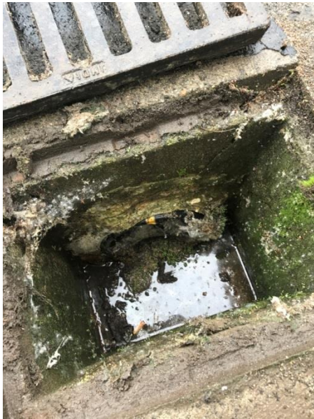
Figure 6. CB5 with lid removed.
